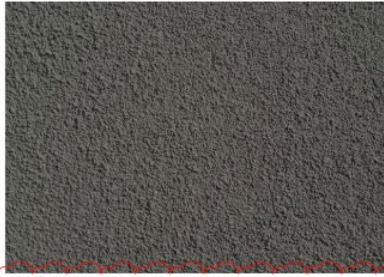
RENDERED BRICK (BK/R) PAINT TO RENDER (DULUX WEATHERSHIELD RENDER REFRESH - COLOUR: RAKU)
